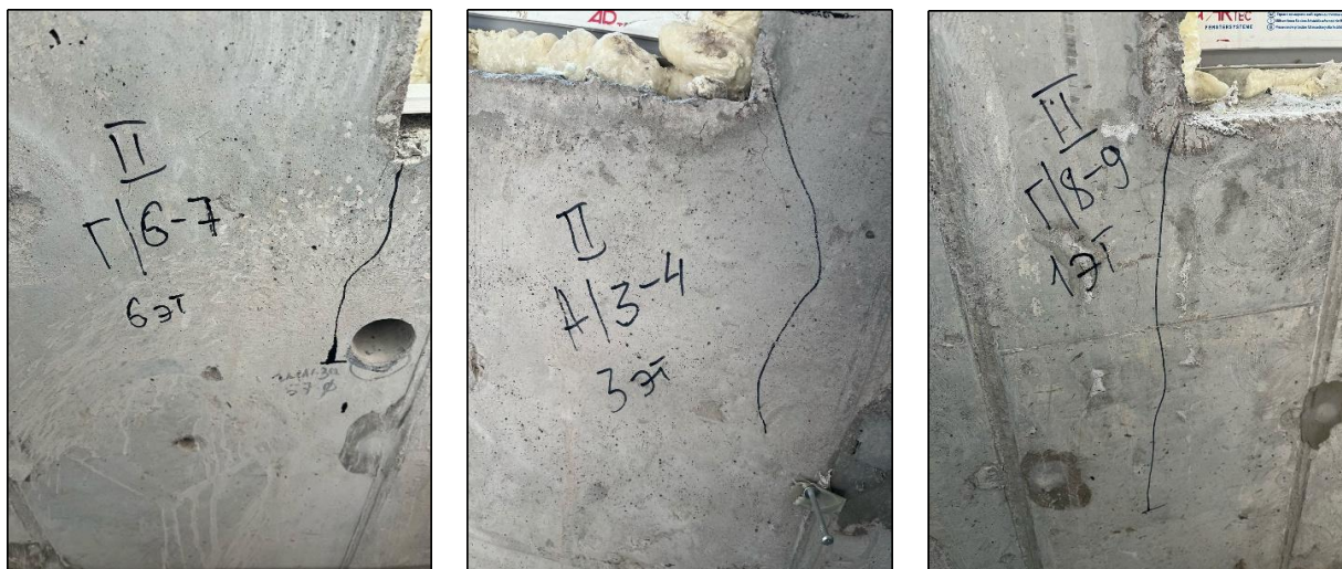
Figure 14. Small hairline cracks developing from the corners of window openings after stage II.
