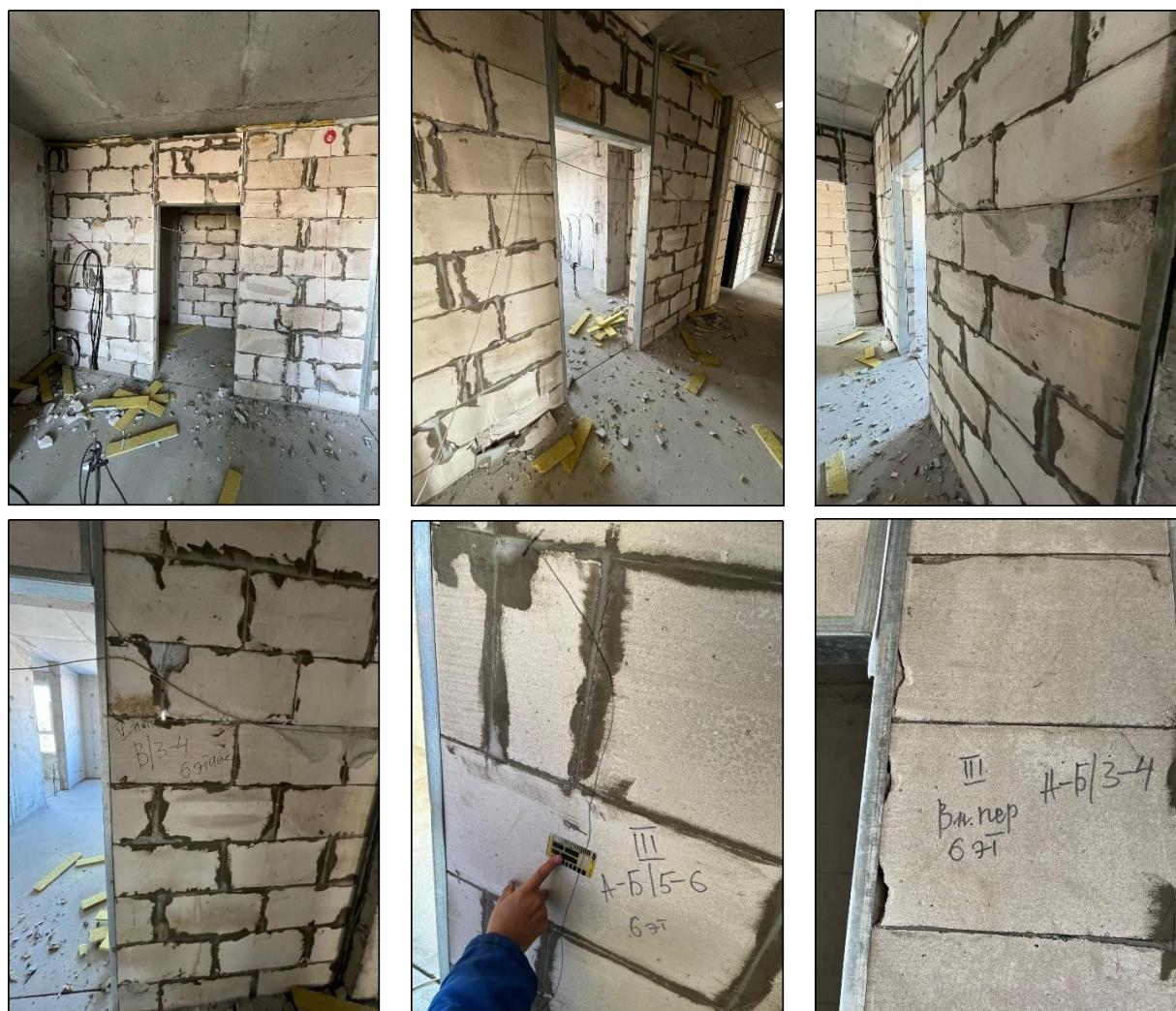
Figure 15. Damage to partitions at the junctions with the floor.
