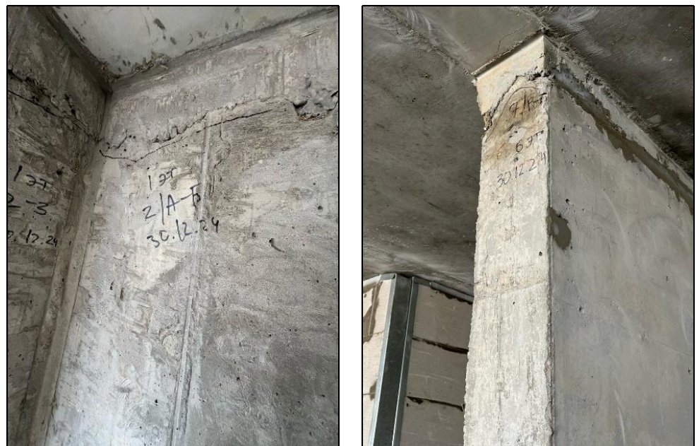
Figure 6. Concrete sag at the floor and roof level.
