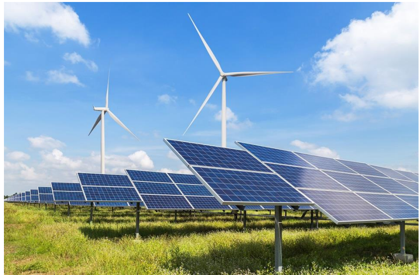
Figure 5. The Keele renewable generator equipment shows the two small wind turbines generating 2 MW, plus the solar panel array contributing 4.4 MW.
