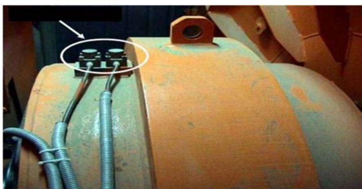
Figure 5. Location of installing acceleration sensors on the bearing housing.
