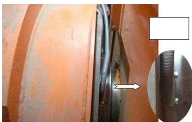
Figure 6. Location of installing displacement sensors on the bearing housing.
