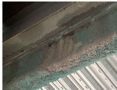
Figure 11. This fireproofing on the beam had already been patched (the light areas). It is in the process of sloughing off again as water leaks onto it – notice the exposed steel.
