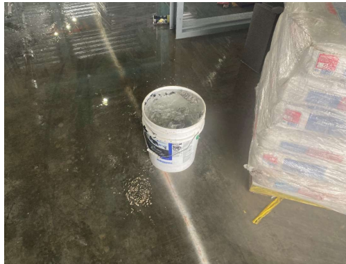
Figure 16. This bucket was placed under a leak. Eventually it filled up and overflowed.
