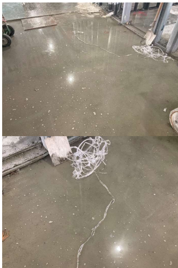
Figure 15. Poor working conditions due to wet floors. This is several floors below roof level.
