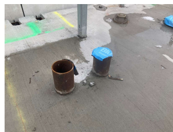
Figure 5. At some point the seal on this sleeve was opened but no one closed it back up.
