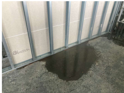
Figure 8. This was on the 1st floor of a six-story building. This drywall ultimately had to be replaced.
