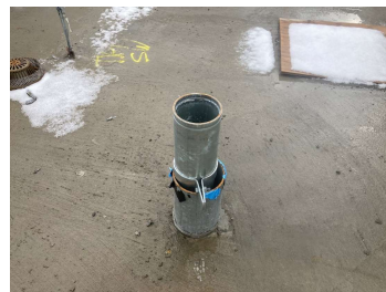
Figure 1. Vent pipe positioned in a roof sleeve. The pipe is not sealed nor is the gap between the sleeve and the pipe.
