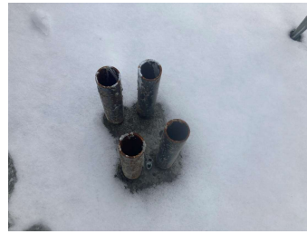
Figure 3. These four penetrations were never sealed.
