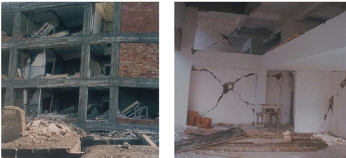
Figure 2. Damage and collapse of illiterately constructed non-load-bearing walls in frame buildings.
