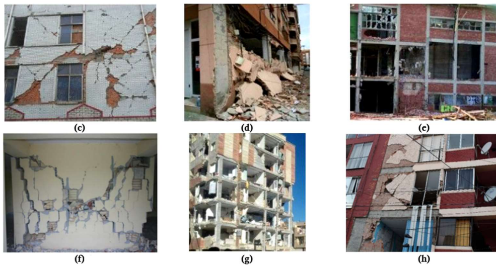
Figure 3. Examples of destruction of the infill walls in frame buildings during earthquakes in different countries. (a) Portugal; (b) Italy; (c) China; (d) Spain; (e) New Zealand; (f) Nepal; (g) Iran; (h) Mexico.
