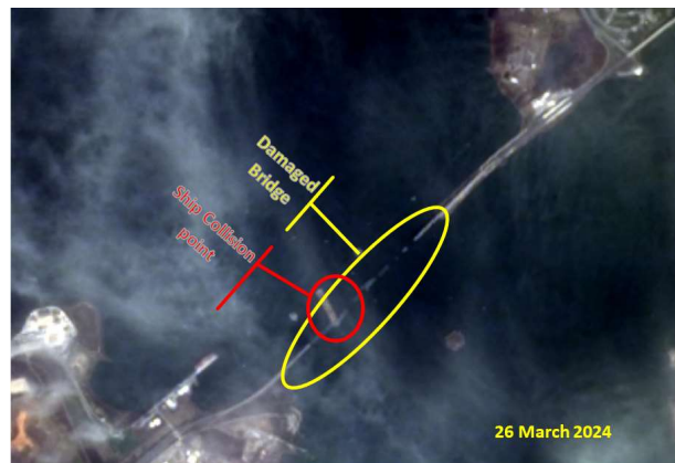
Figure 5. 26 March 2024—Post collision.
