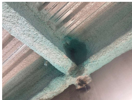
Figure 12. Water penetrating the fireproofing as it started to rain.
