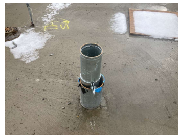
Figure 1. Vent pipe positioned in a roof sleeve. The pipe is not sealed nor is the gap between the sleeve and the pipe.
