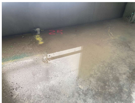
Figure 17. This building has precast concrete wall panels. Water is running off the floor slab and falling down between the gap to lower floors.
