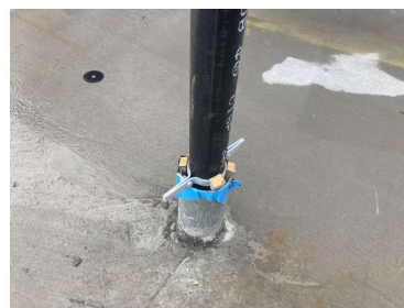
Figure 2. Temporary sleeve seal was breached by the pipe and not resealed.
