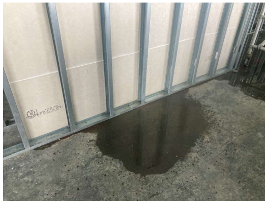
Figure 8. This was on the 1st floor of a six-story building. This drywall ultimately had to be replaced.
