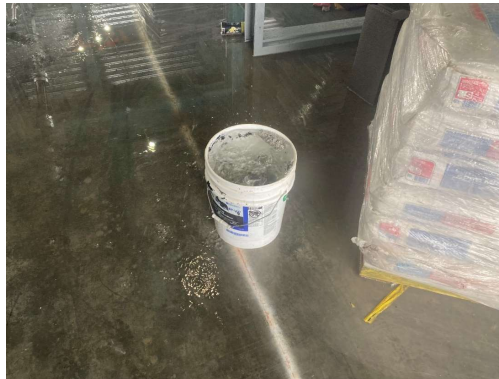
Figure 16. This bucket was placed under a leak. Eventually it filled up and overflowed.
