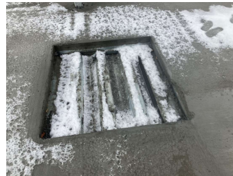
Figure 4. An alternative to leaving a large penetration is to place the metal decking but not pour over it.
