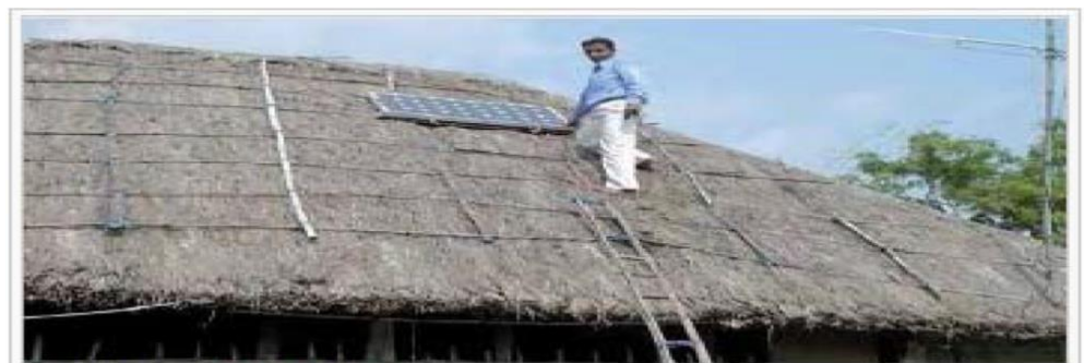
Figure 6. Solar panel on the roof top in Sub-Saharan African remote area [20,22].
